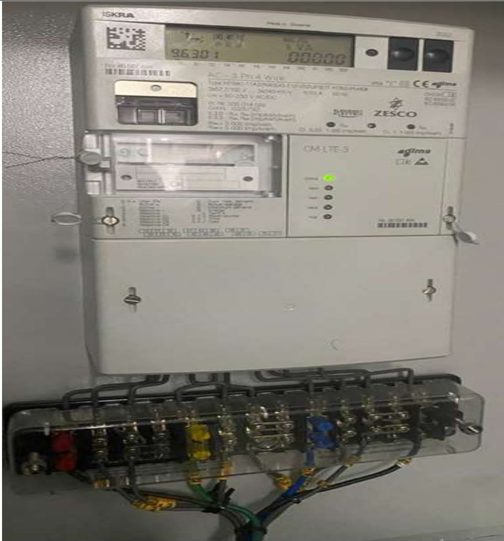
Fig. 4. Three phase meter at 66/11kV Depot substation (source: field data 2024).
